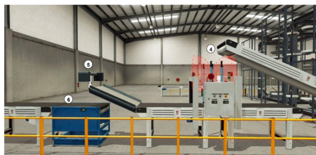
Figure 7: Finishing of the process: sensors, camera, winding and automatic balance.
