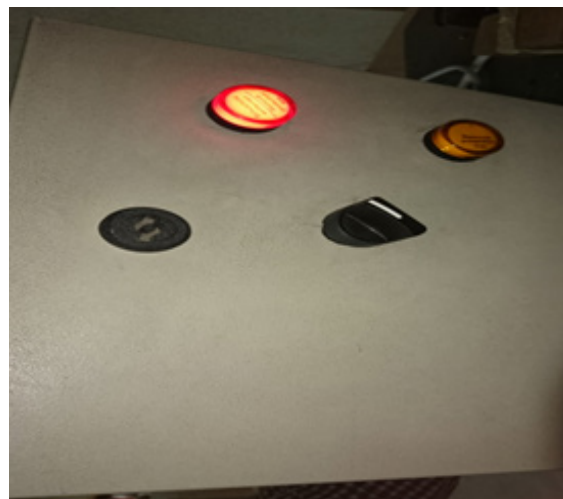
Figure 15: On hand/ manual mode, The system is working.
