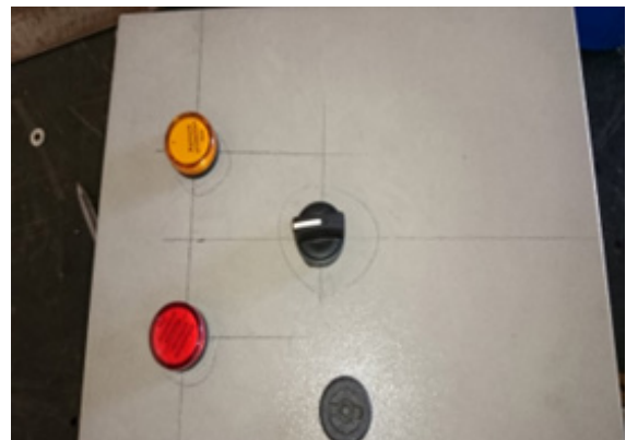
Figure 9: Indication lights and selector switch inserted in its positions.
