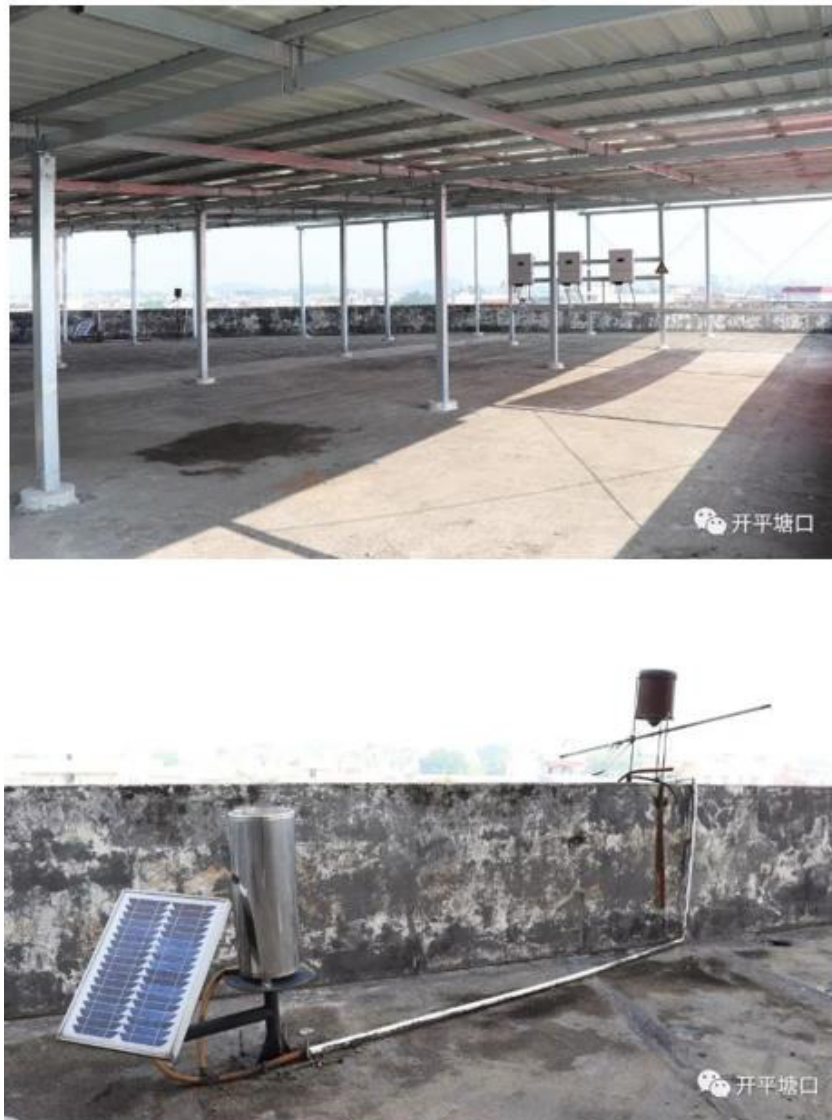
Figure 1: Photovoltaic power station.
