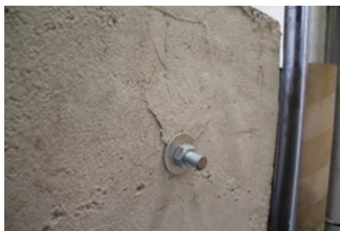
Figure 4e: Some cracks are only associated with the anchoring point and terminate before reaching the side edge of the element. The crack has been graphically redrawn. In most cases, the load tests ended with surface or structural damage to the concrete as a result of exceeding the bearing capacity in compression.
