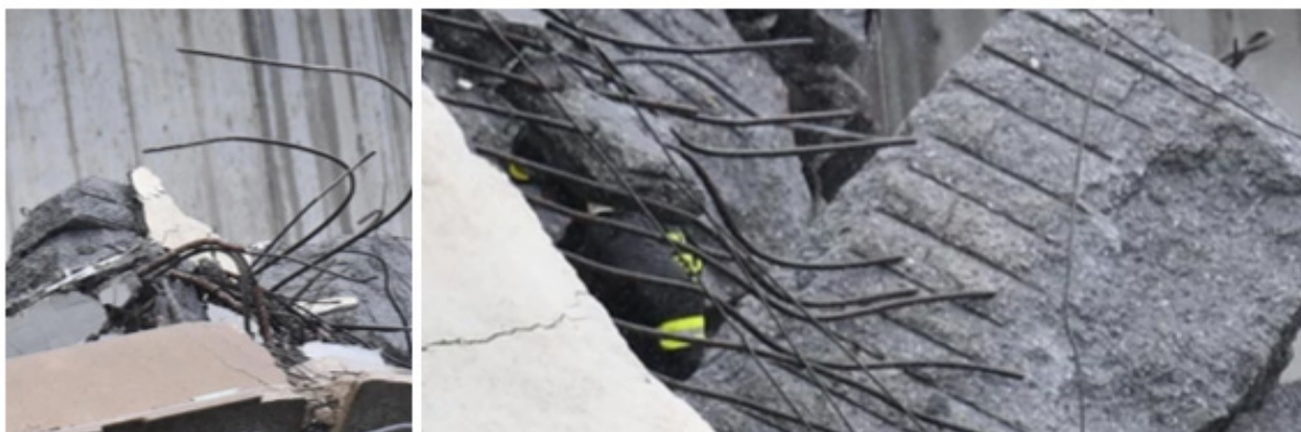
Figure 5: Reinforcement of a collapsed bridge in Genoa with visible ruptures of steel prestressing tendons [own study].
