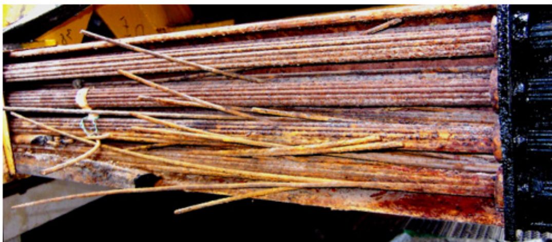
Figure 3: Example of damage to girder prestressing tendons [own study].
