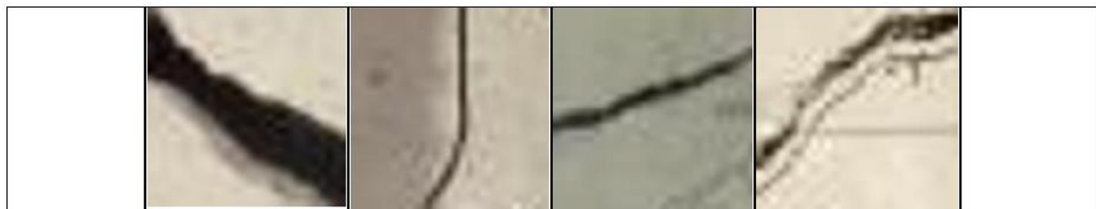
Figure 12: Example of crack images.
