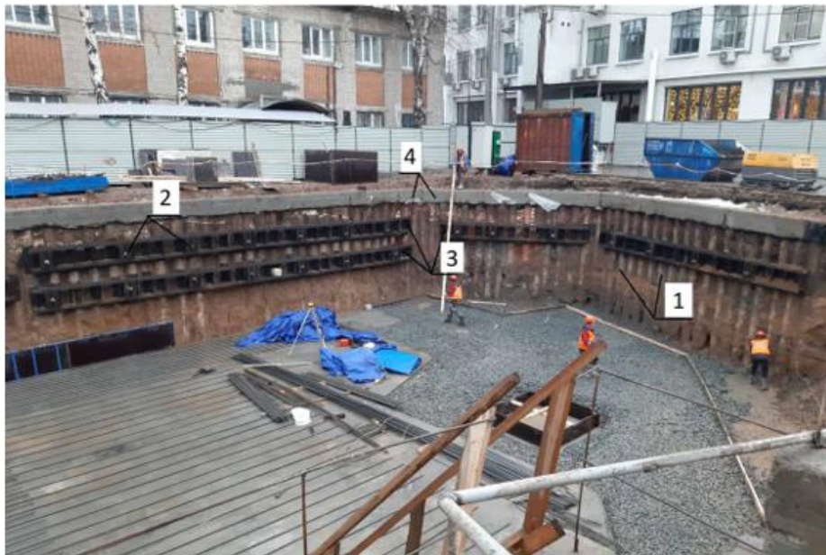
Figure 6B: Fragment of the pit fencing plan: 1-boroinjective ERT piles; 2-ground ERT anchors; 3-anchor strapping belt; 4-monolithic reinforced concrete strapping belt.
