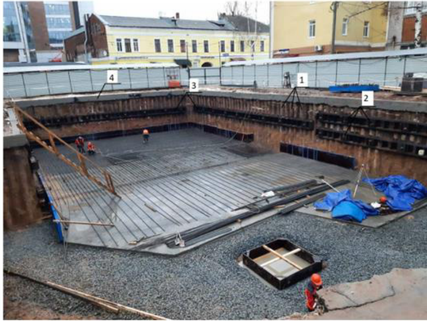
Figure 6A: Fragment of the pit fencing plan: 1-boroinjective ERT piles; 2-ground ERT anchors; 3-anchor strapping belt; 4-monolithic reinforced concrete strapping belt.
