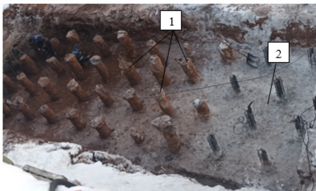
Figure 2: Pile field for a monolithic reinforced concrete buttress: 1-heads of EDT bored injection piles; 2-concrete preparation for grillage.
