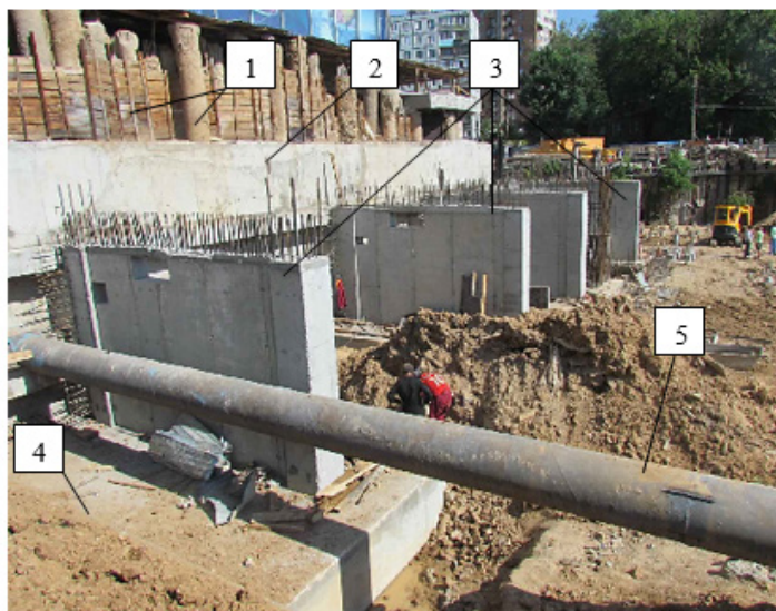
Figure 3: Fragments of the completed monolithic reinforced concrete buttresses: 1-existing bored piles to enclose the excavation; 2-fencing of the pit from monolithic reinforced concrete; 3-monolithic reinforced concrete buttresses to reinforce the existing retaining wall; 4-monolithic reinforced concrete grillage; 5-existing pipe - amplification shooting.
