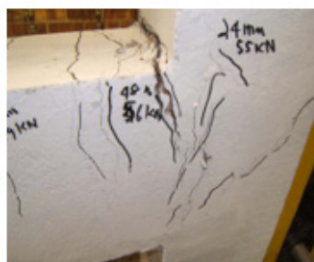
Figure 18: Beam-column joint with SFRC 1st / 2nd / 3rd cycle.
