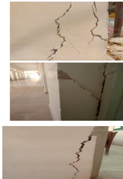
Figure 2: Cracks showing size and orientations in the building.
