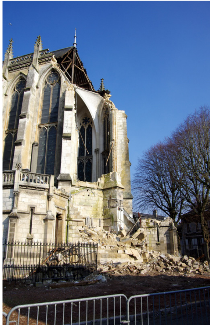
Figure 4: Liability or resource? Case in point: Victor Delefortrie, Saint-Jacques, Abbeville, France 1868– 1876, demolished 2013, photo: Marc Roussel (CC BY-SA 3.0).
