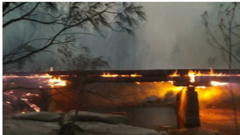
Figure 2: Mann River Bridge, Wyaliba on fire, 8 November 2019 [2].
