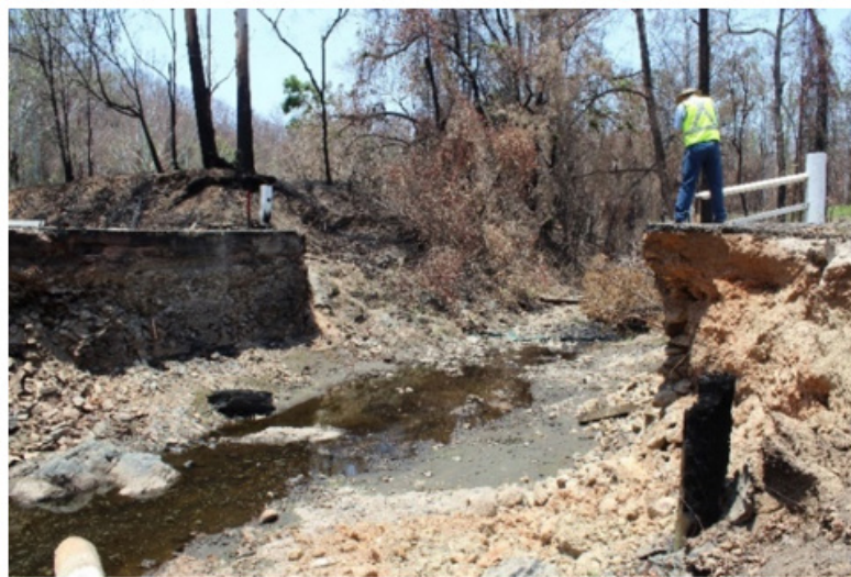
Figure 6: Hortons Creek bridge site, with fire-damaged timber removed (Glencross-Grant, 2 January 2020).
