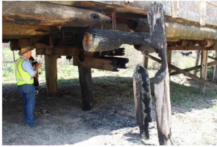
Figure 4: Fire-damaged Clouds Creek Bridge, showing destroyed outer pile, corbel, ends of girders and headstock highlighting end grain progression (Glencross-Grant, 2 January 2020).
