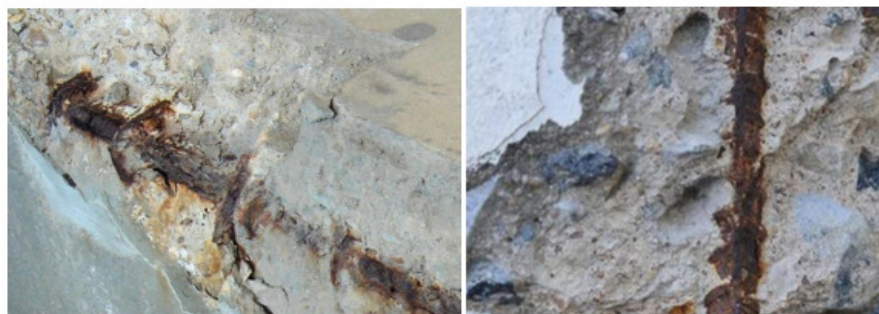
Figure 2: Corrosion of reinforcement due to carbonation of concrete.
