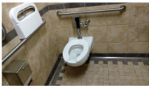
Figure 3: Water efficient toilet. Courtesy: NC A&T State University.
