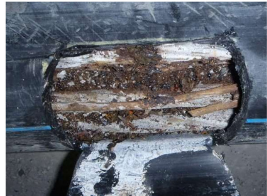
Figure 1: An example of deteriorated tendon in post-tensioned bridges.
