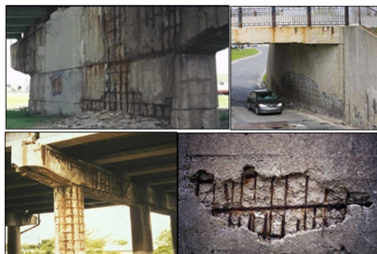
Figure 1: Corrosion of reinforced concrete structural elements.
