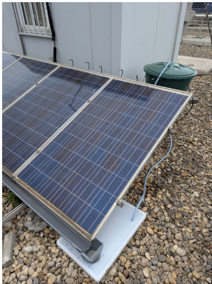
Figure 2: Facility installed in the Bilbao School of Engineering.
