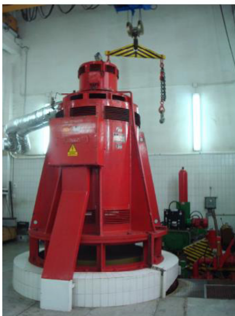
Figure 6: Picture of the vertical Francis turbine installed until 2016.
