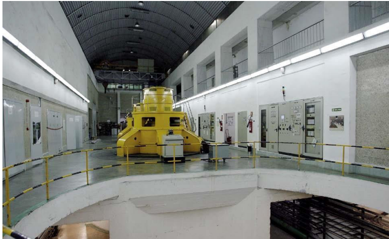
Figure 2: Photograph of one of the generators connected to the corresponding Francis turbine in Barazar HPP.
