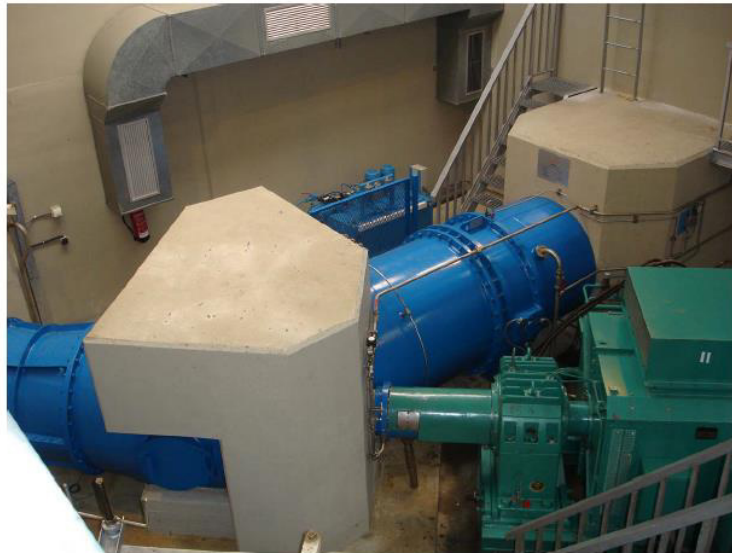
Figure 3: Photograph of one of the turbines installed in Undurraga HPP.
